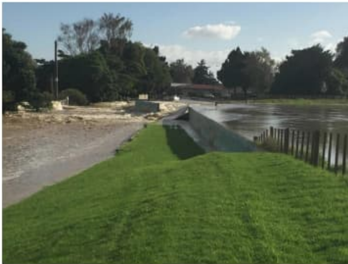
Figure 3.3: (Caption taken from report) The breached Floodwall at Edgcombe, looking downstream; image file, date stamped 0835 6th April, some 5 minutes after the breach (Source: BOPRC Contractor, 2017).
