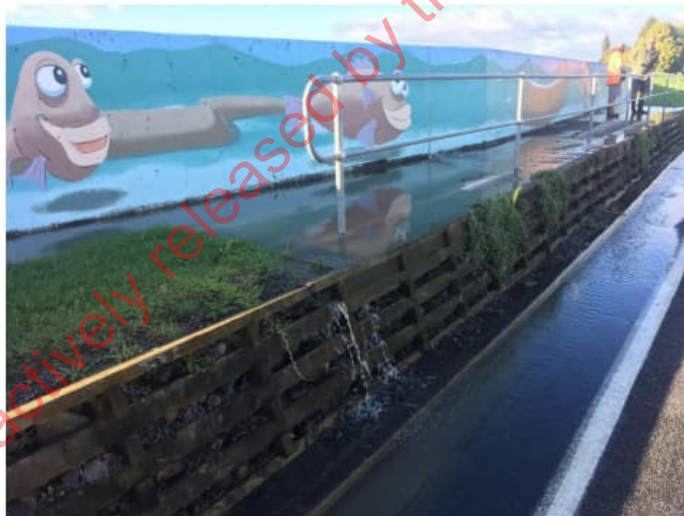
Figure 3.2: (Caption taken from report) The Edgecumbe Floodwall, known locally as 'The Painted Wall', at 0814 on 6th April, 15-20 minutes before the breach (Source: BOPRC, 2017)
