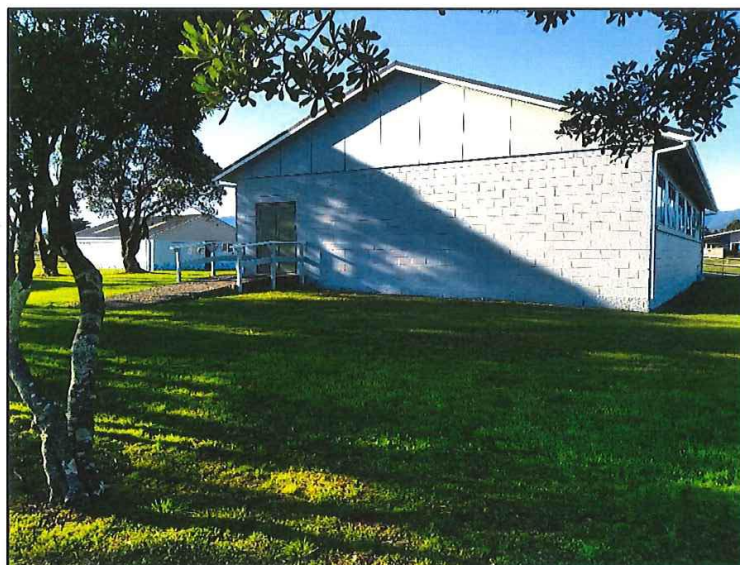
Carters Beach Hall; freshly painted but requiring seismic strengthening on the seaward wall
